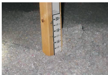
Figure 213-3-1-2: Attic insulation marker
