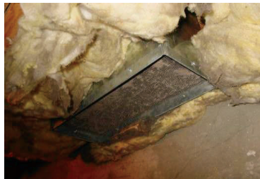
Figure 311-3-2: Dirty combustion air intake to wood stove that needs to be cleaned
