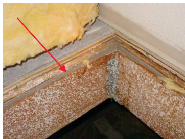
Figure 215-3-1: Peel & stick weatherstripping is not permitted
