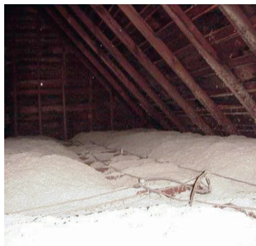
Figure 213-1-4: Attic insulation installed under knob-and-tube wiring
