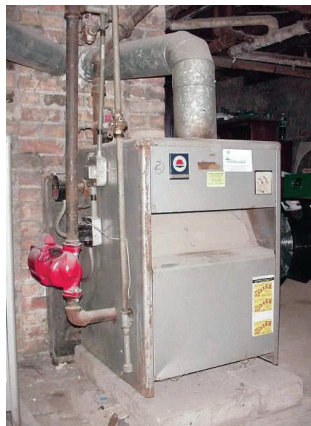
Figure 316-1-1: Warm water boiler
