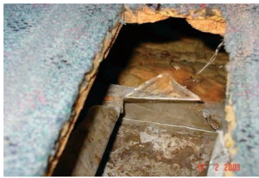
Figure 411-4-1: Opening between duct boot and floor
