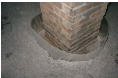
Figure 213-1-3: Metal barrier around chimney
