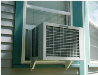
Figure 315-6-1: Room air conditioner
