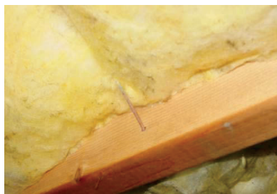
Figure 215-2-3: Compressed insulation due to insulation support
