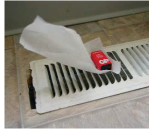
Figure 114-1-3: Sometimes duct leakage is obvious before you use the pressure pan; air coming
