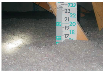
Figure 213-8-1: Attic insulation marker
