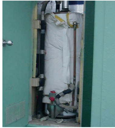
Figure 412-1: Existing mobile home water heater
