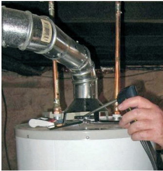
Figure 312-3-1: CO reading taken for water heater before dilution air
