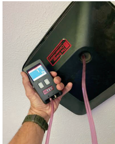
Figure 114-2-1: Tight duct measuring 1.1 Pa
