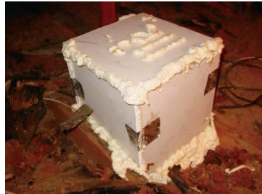
Figure 213-1-1: Recessed light covered with drywall box
