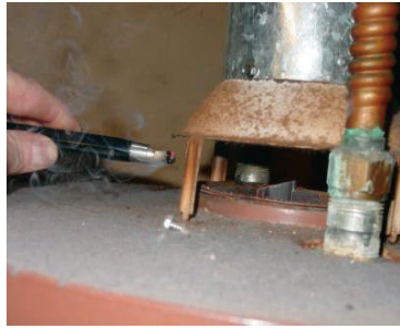
Figure 117-2: Failed spillage test
