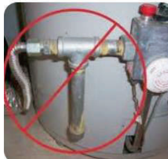
Figure 319-2-2: Incorrectly installed sediment trap
