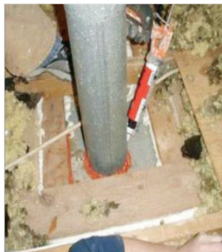
Figure 213-1-2: Metal barrier around flue sealed with high temperature caulk
