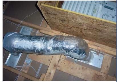
Figure 115-3-1: Jumper duct installed in attic connecting bedroom to hallway (Courtesy Southface Institute)
