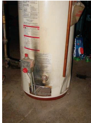
Figure 311-1-1-1: Evidence of flame roll-out
