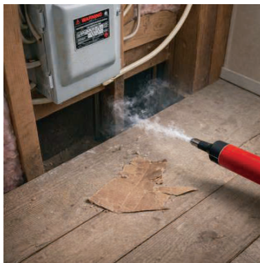
Figure 212-1-1: Smoke being drawn down an open stud cavity indicating leakage to the inside
