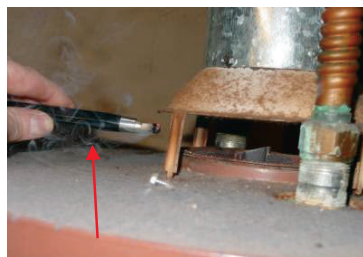
Figure 312-2-2: Appliance fails spillage test
