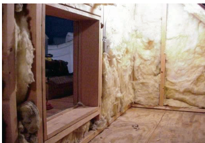
Figure 213-6-4-1: Knee walls insulated with fiberglass insulation
